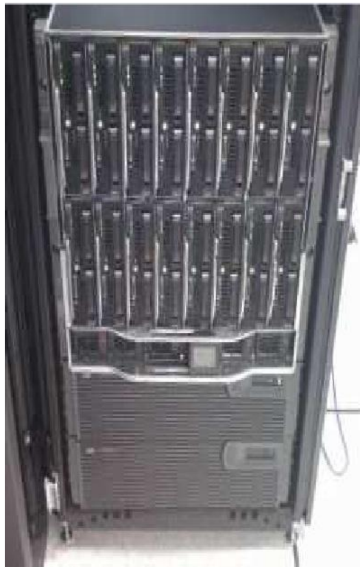
HP Blade System c7000 enclosure (populated with 16 blades), with two 3U UPS units below
