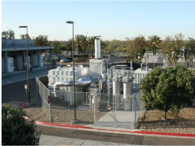
1.4 MW DFC1500 at a municipal facility
